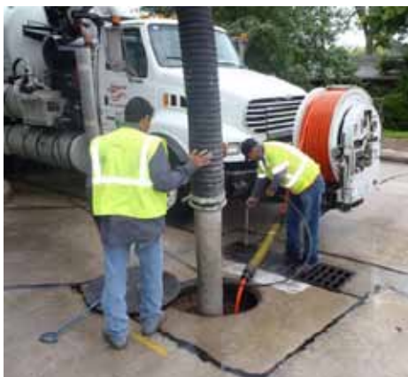
On an annual basis, crews jet and vacuum storm drain lines and inlets to alleviate potential flooding and reduce harmful pollutants.
